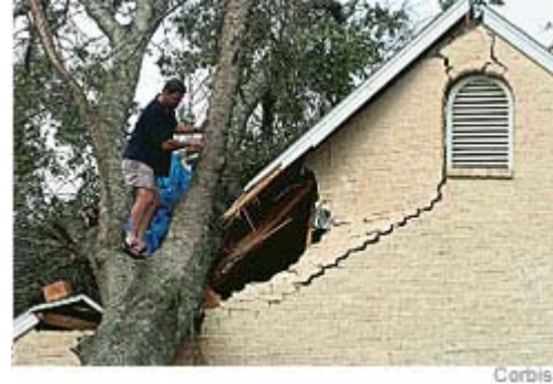
A house in Lake Charles, La., with roof damage after Hurricane Rita.
